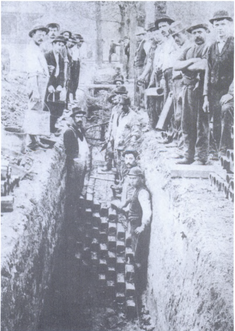
Fig. 18. Laying Telephone Conduits Underground. (Herbert N. Casson, The History of the Telephone , Chicago: A. C. McClurg and Co., 1911, f. 238)
